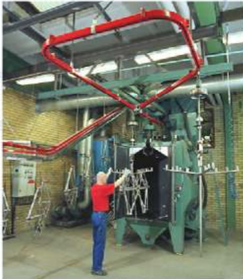
Loading, unloading area to a shot blasting machine
